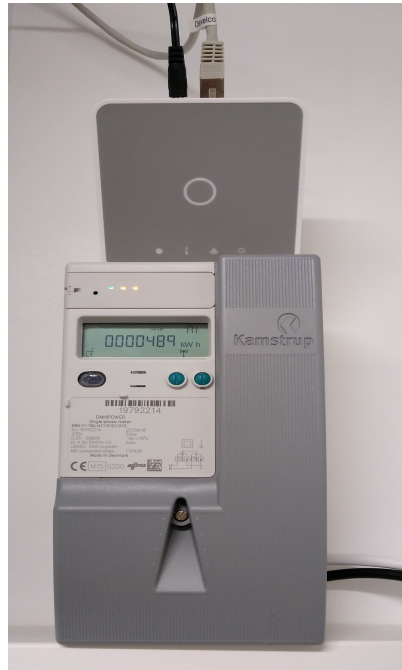
Figure 10. Kamstrup Smart meter.
